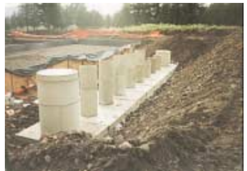
Pump chambers for recirculating sand filter Yellowstone National Park
