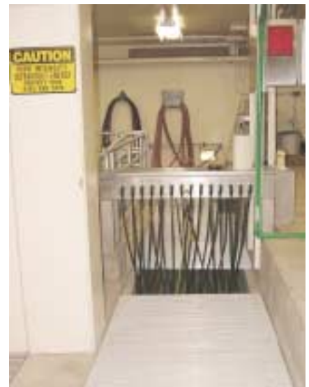
Ultraviolet Disinfection is Often the Best Approach for High-Quality Effluents.
