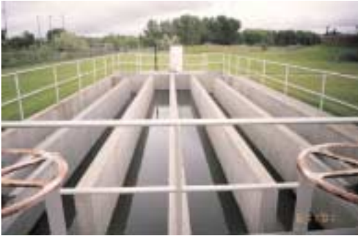
Chlorine Contact Basin
